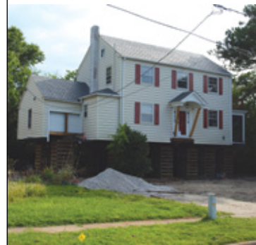
▲ FIGURE 1. In Norfolk, VA, homeowners raise their houses by up to 8 feet to be pro- tected against the nuisance flooding.
